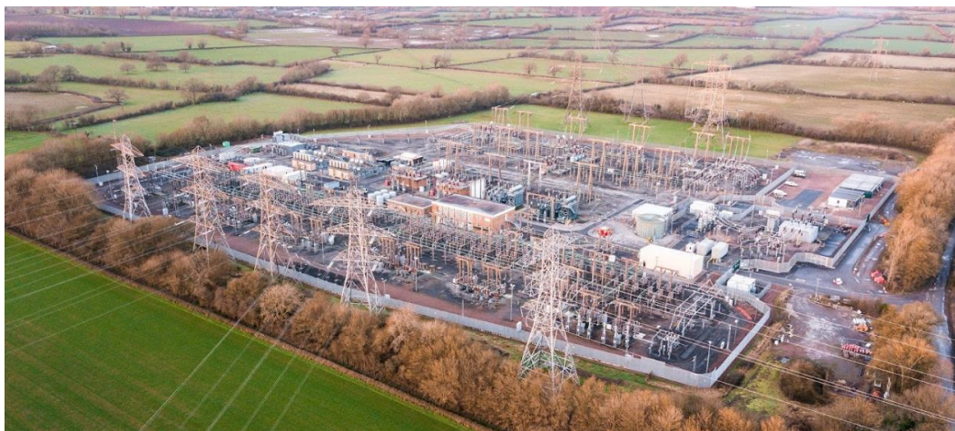
Iron Acton substation. (James Williams – Google Maps)
