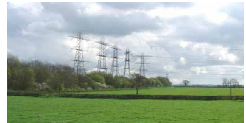
8 Pylon towers at Iron Acton electricity sub station.
